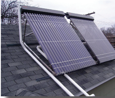
Roof-mounted evacuated tube collectors
